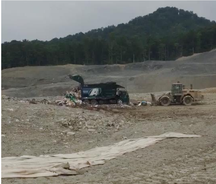
Figure 2. View of typical disposal of waste from a garbage truck at BRLF with a compactor unit about to push waste into waste mass.
