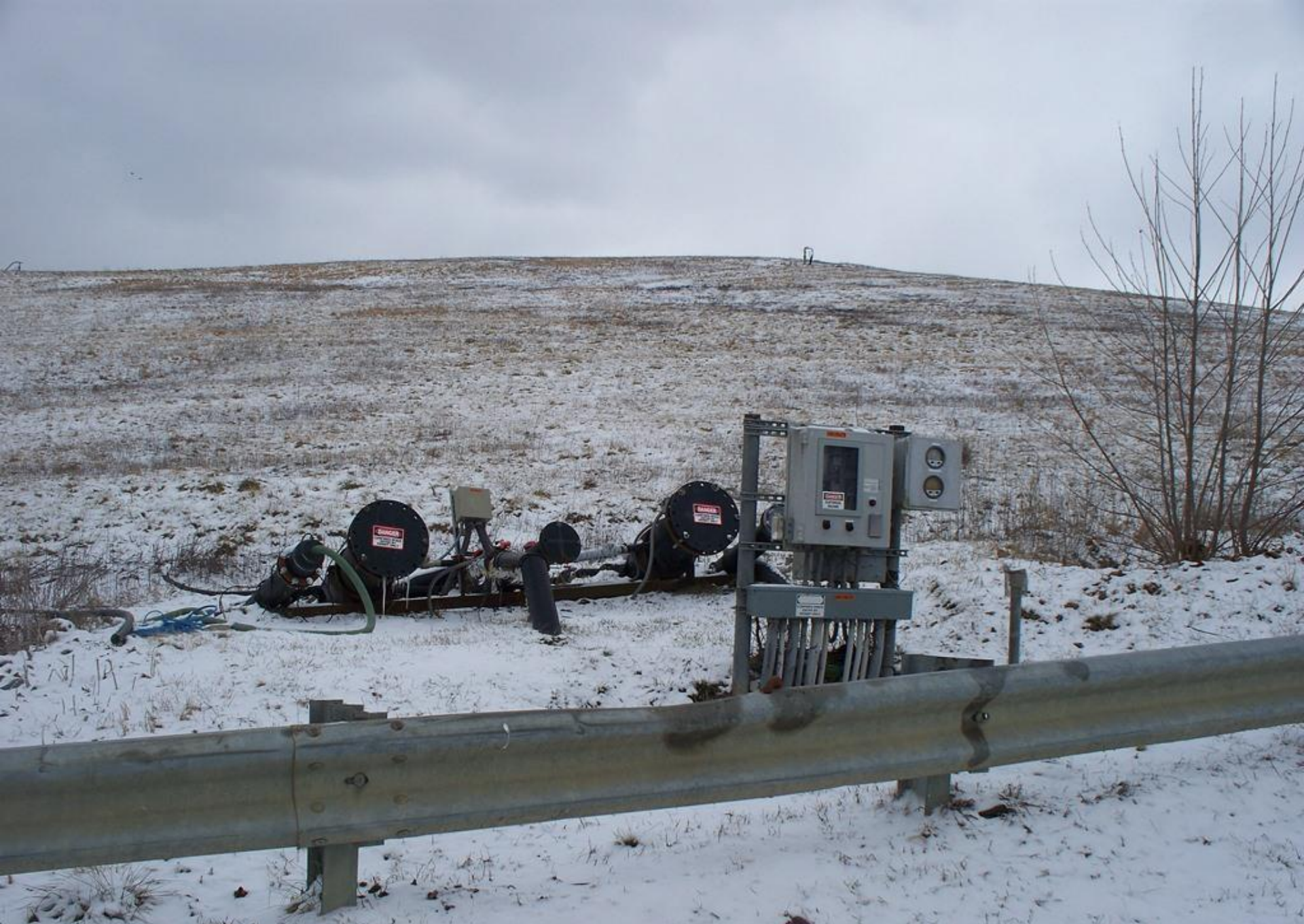
Advanced Disposal Blue Ridge Landfill AI 998 2/10/16 g. weems Landfill water level detector
