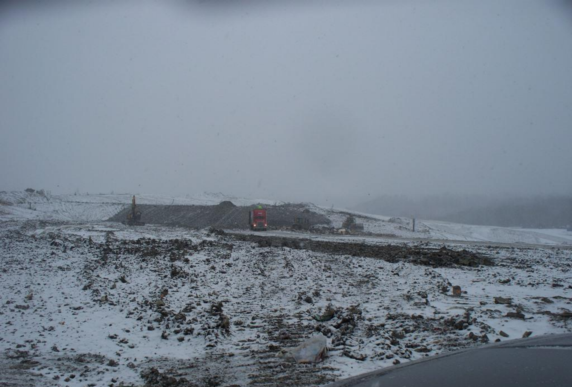
Advanced Disposal Blue Ridge Landfill AI 998 2/10/16 g. weems Working face viewed from solidification pit.
