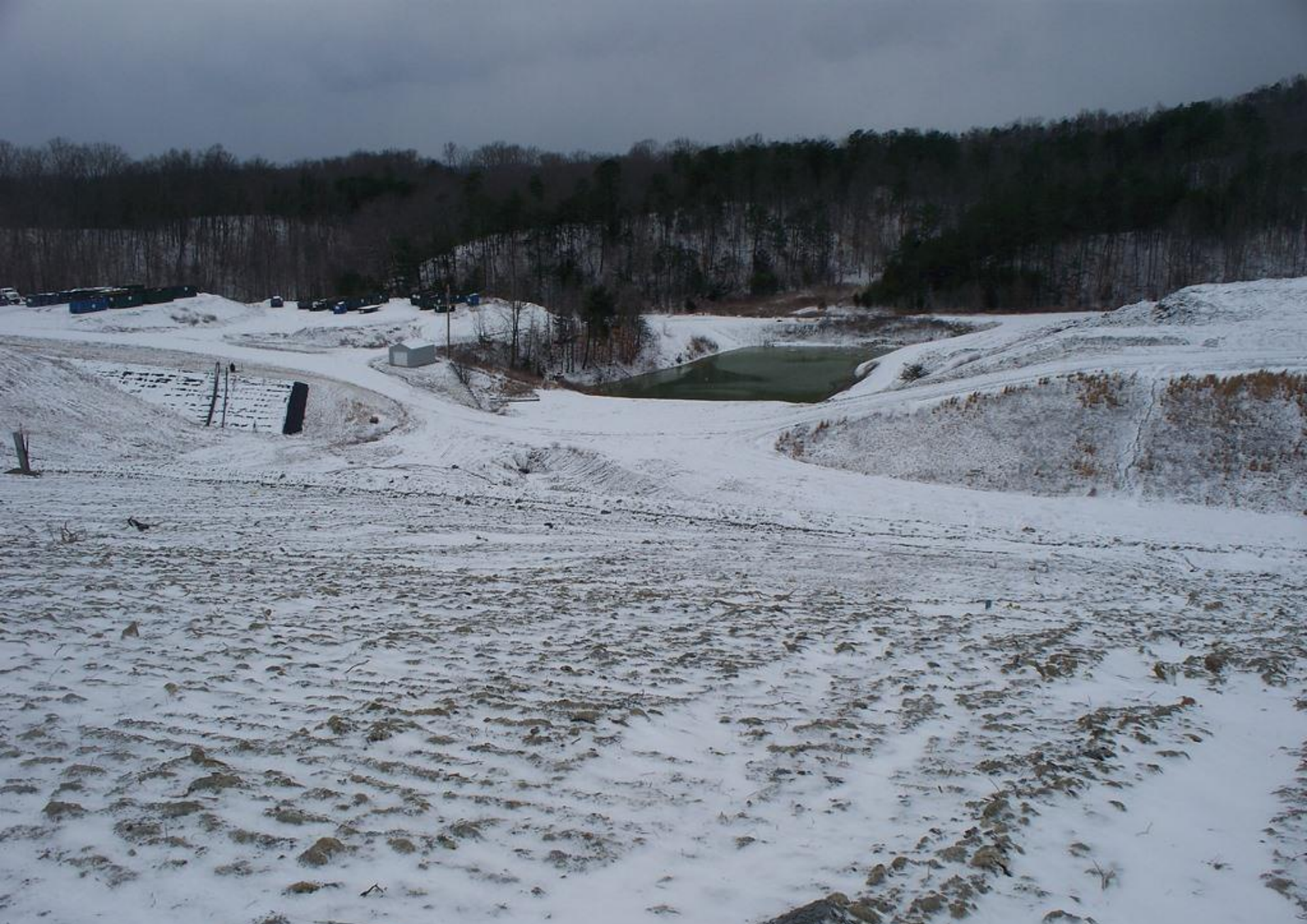
Advanced Disposal Blue Ridge Landfill AI 998 2/10/16 g. weems North side of working face.
