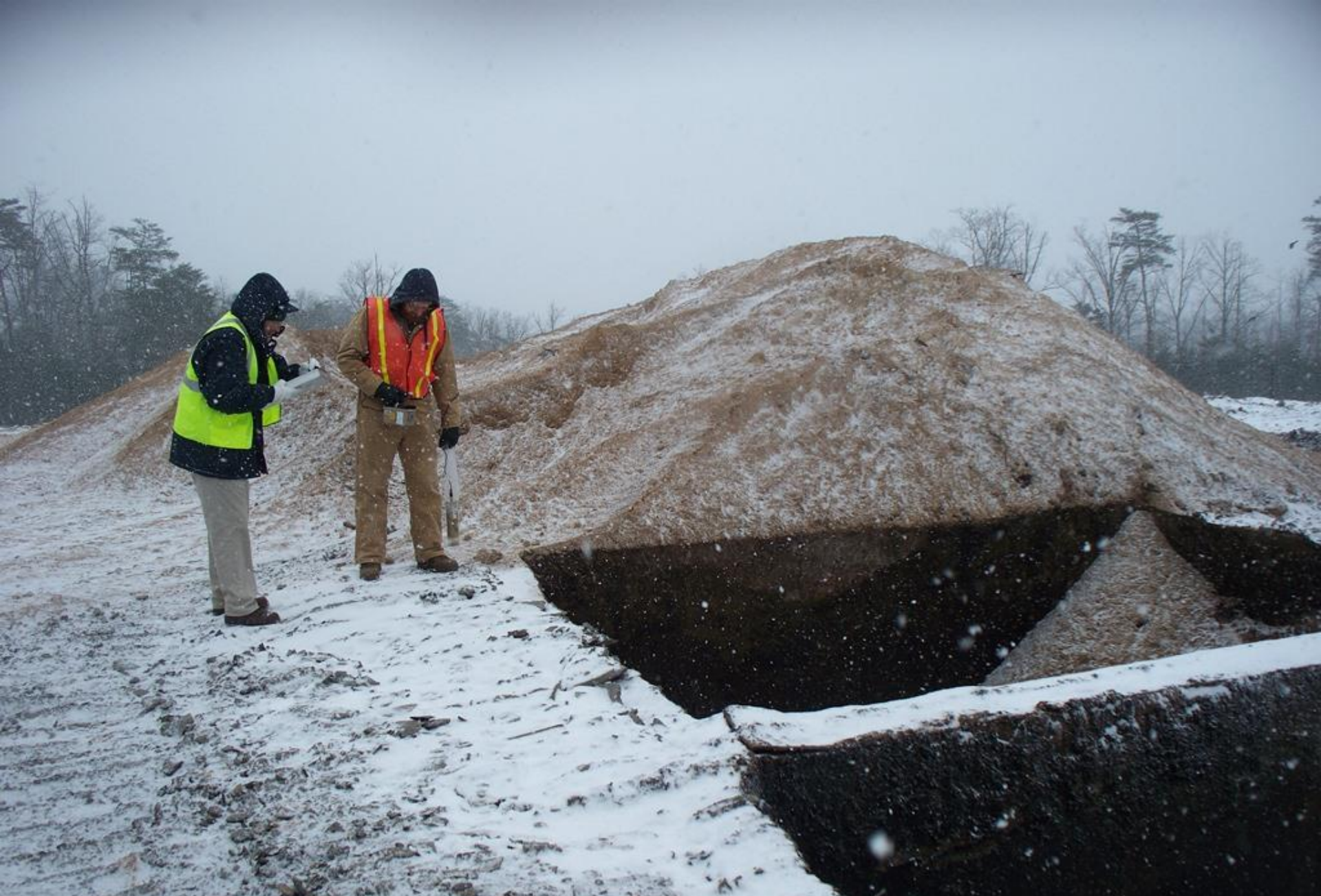
Advanced Disposal Blue Ridge Landfill AI 998 2/10/16 g. weems solidification pit. Testing for TENORM.
