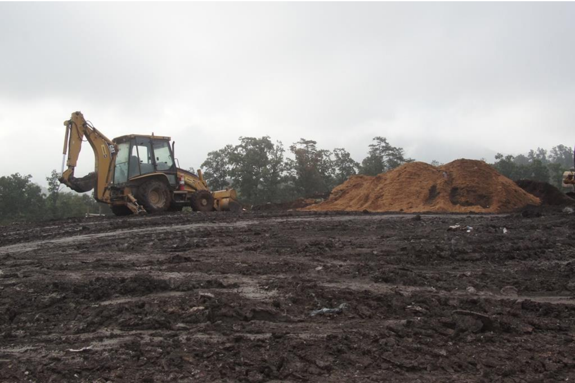
Advanced Disposal Blue Ridge Landfill AI 998 9/11/15 g. weems area for solidifying wet loads.
