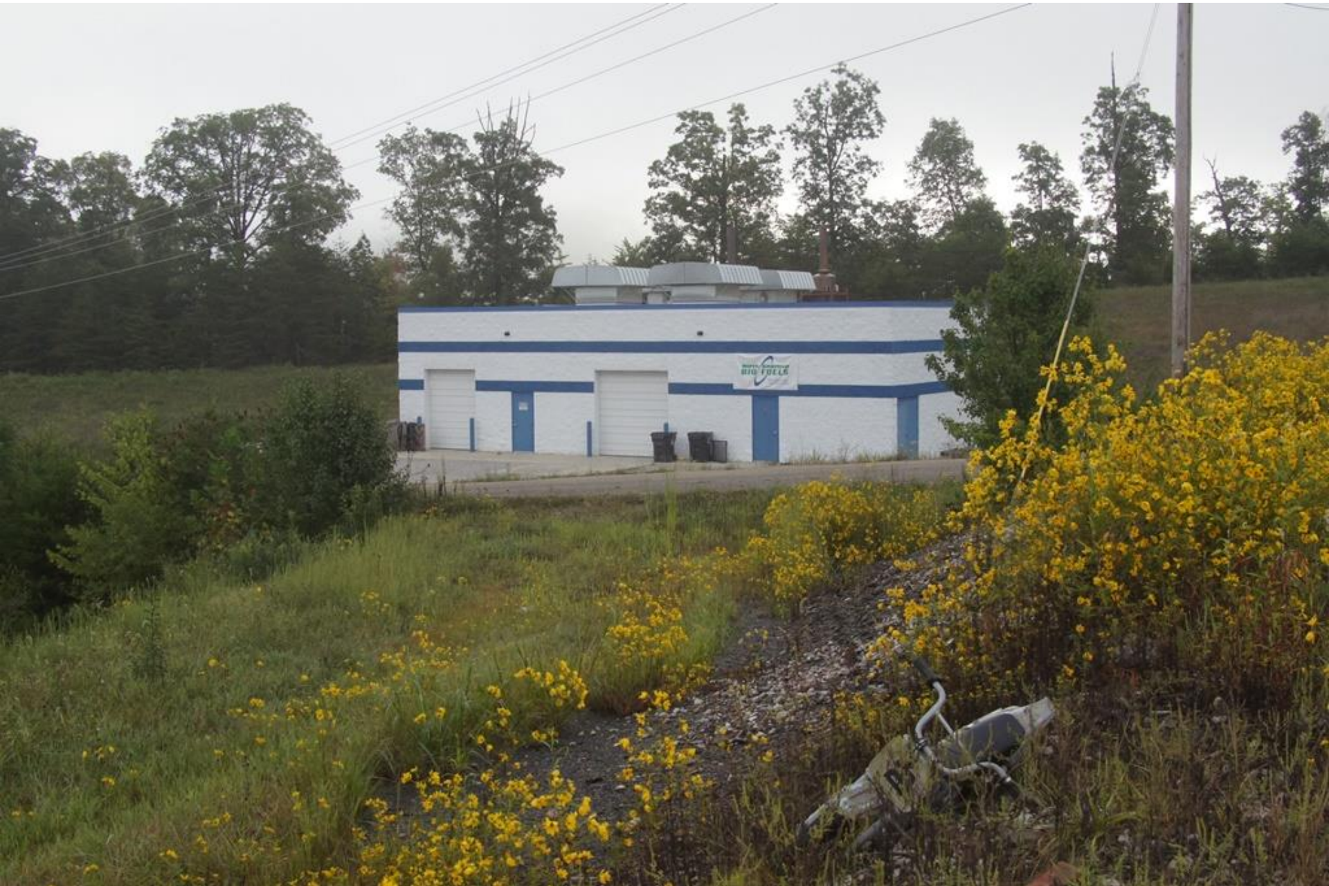
Advanced Disposal Blue Ridge Landfill AI 998 9/11/15 g. weems Landfill gas powered generator
