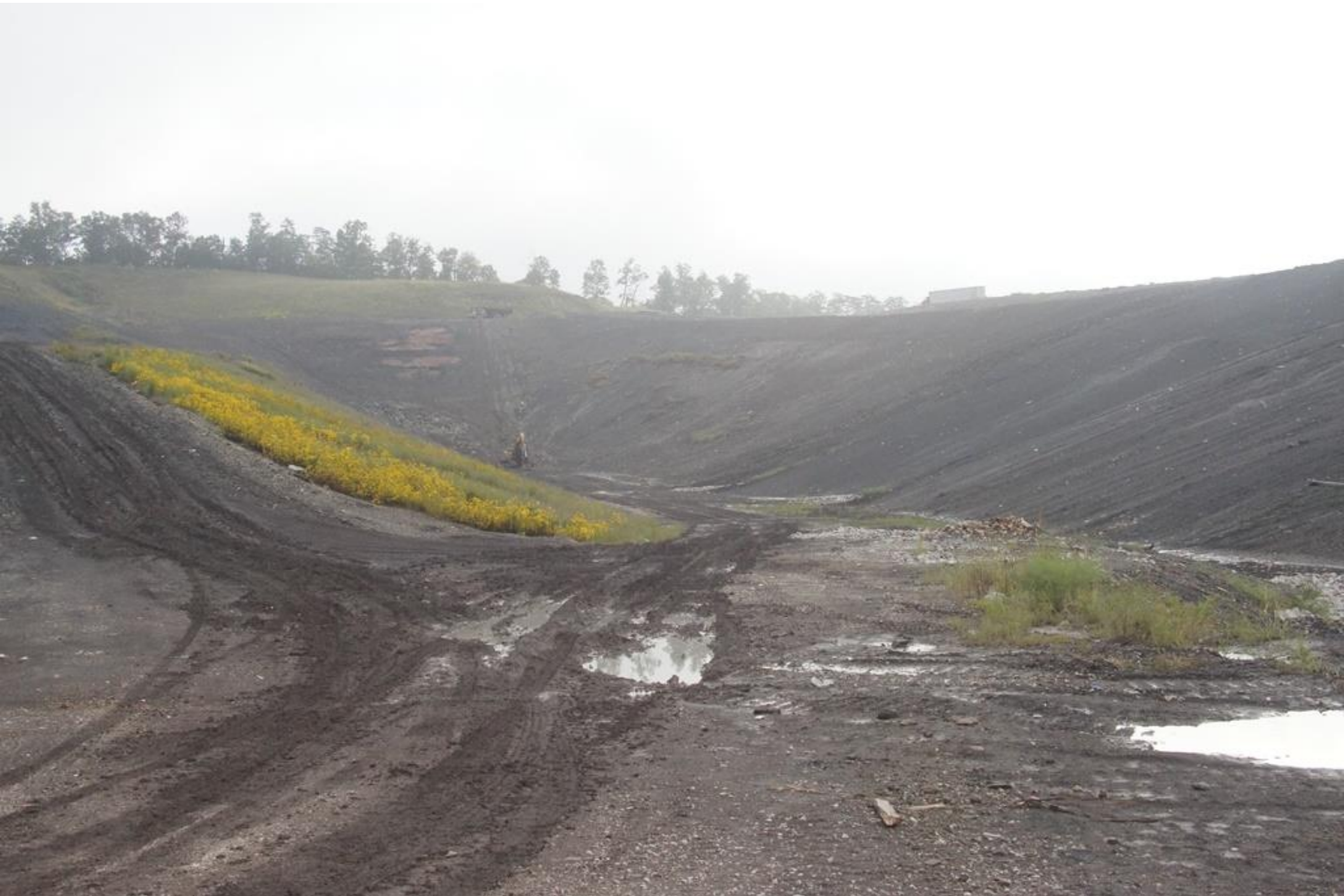
Advanced Disposal Blue Ridge Landfill AI 998 9/11/15 g. weems Even after rain, no leachate outbreaks
