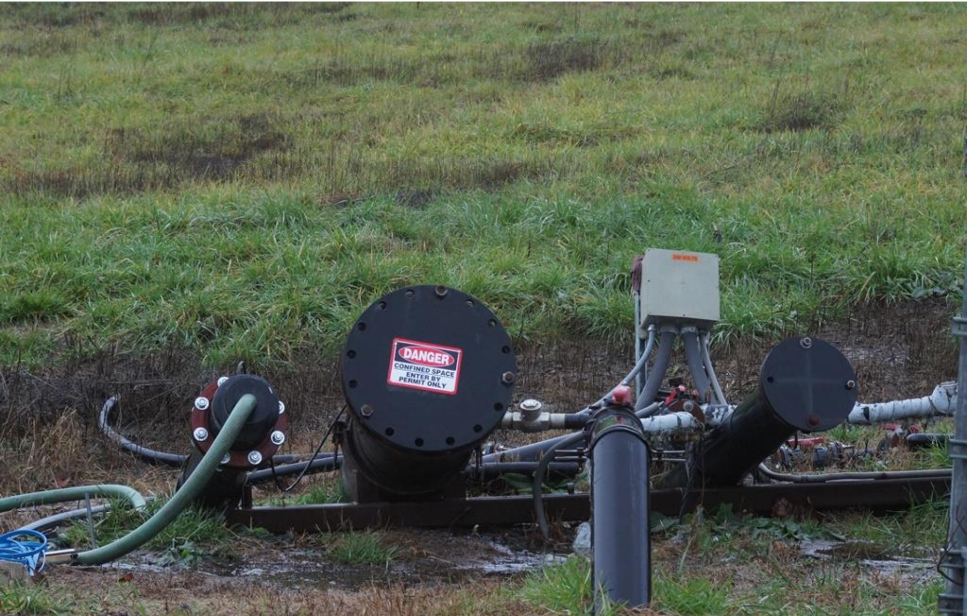
Advanced Disposal Blue Ridge Landfill AI 998 12/1/15 g. weems Bubbler and pumping apparatus at this site. Leachate is pumped to the Irvine WWTP.
