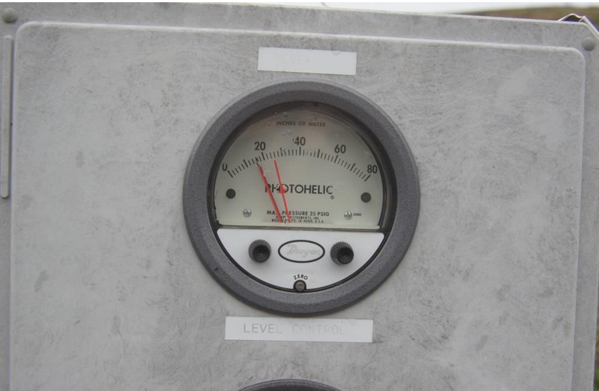
Advanced Disposal Blue Ridge Landfill AI 998 12/1/15 g. weems Bubbler; if water covers tube in landfill, the pressure will rise as water gets deeper.
