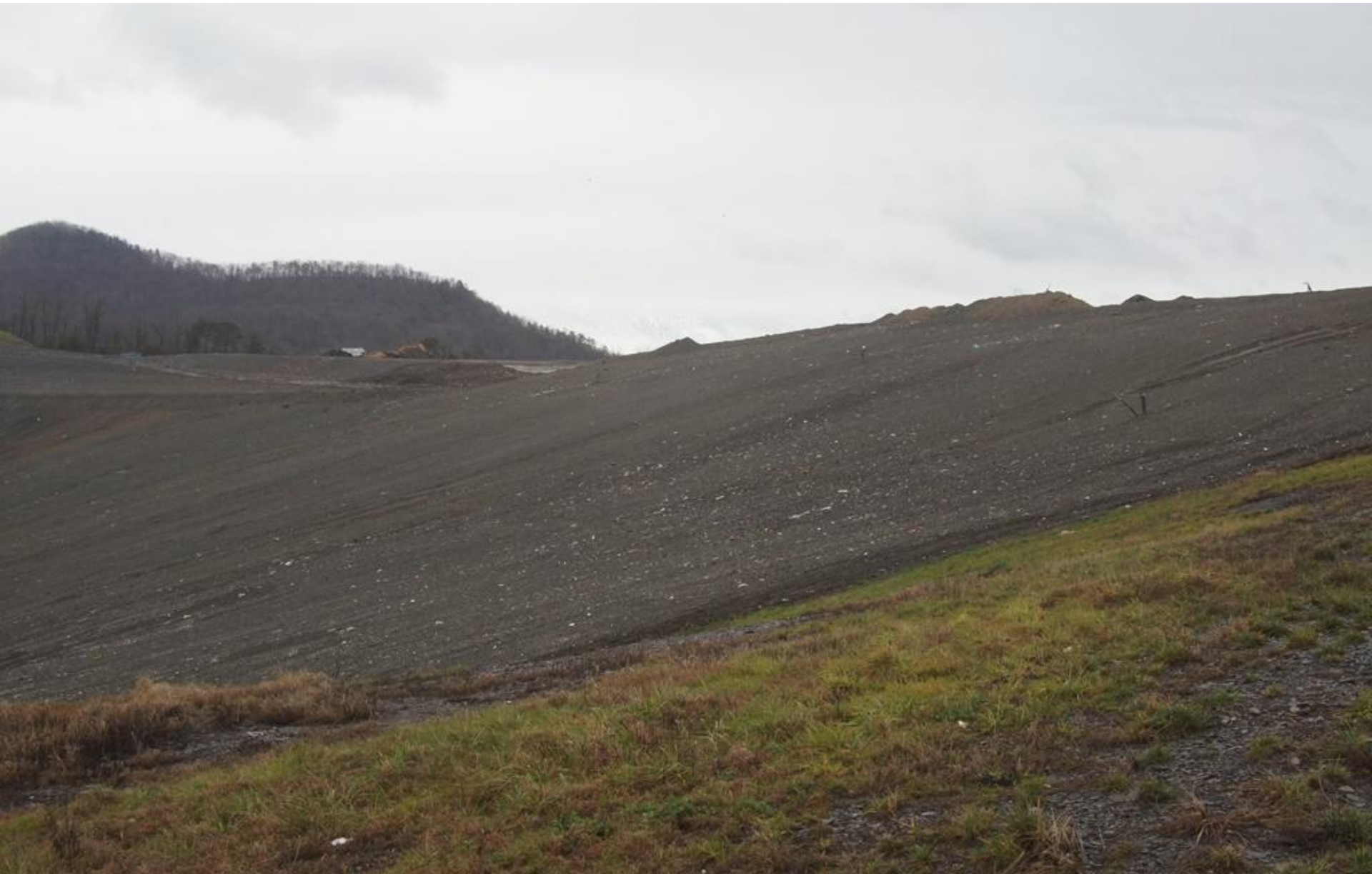
Advanced Disposal Blue Ridge Landfill AI 998 12/1/15 g. weems North side of landfill. No leachate visible; no washing even after heavy rains for two days.
